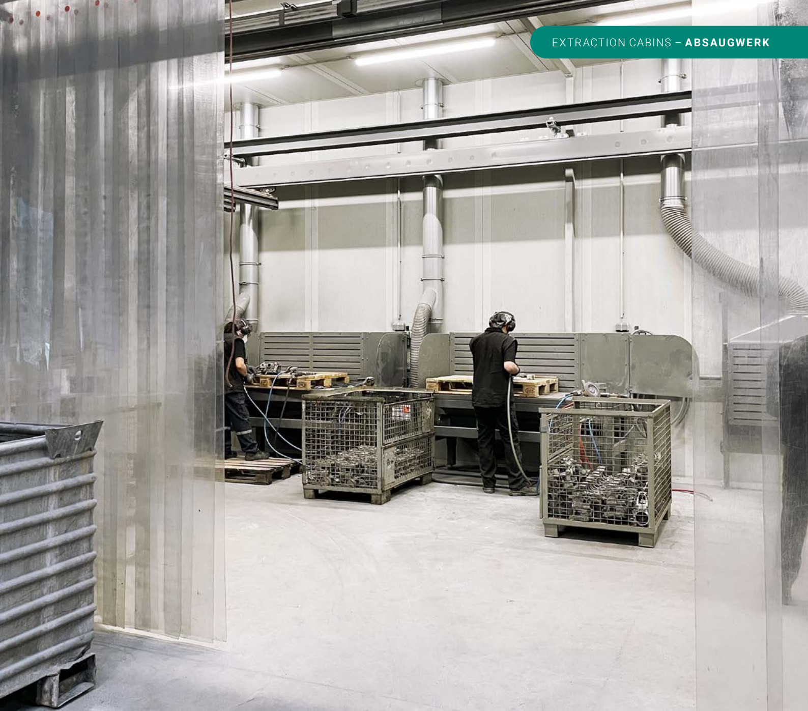
Sound-insulated grinding cabin with integrated extraction tables for safe capture of explosive aluminum dust (ATEX)
